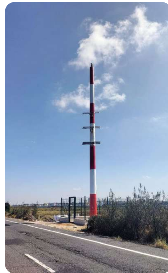
Camera installed on the dyke road.
