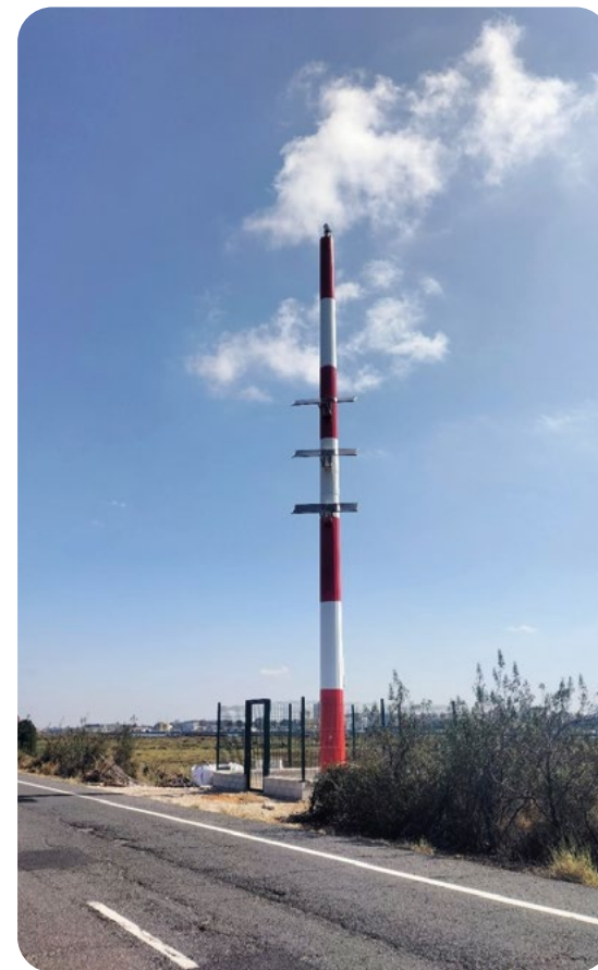
Camera installed on the dyke road.
