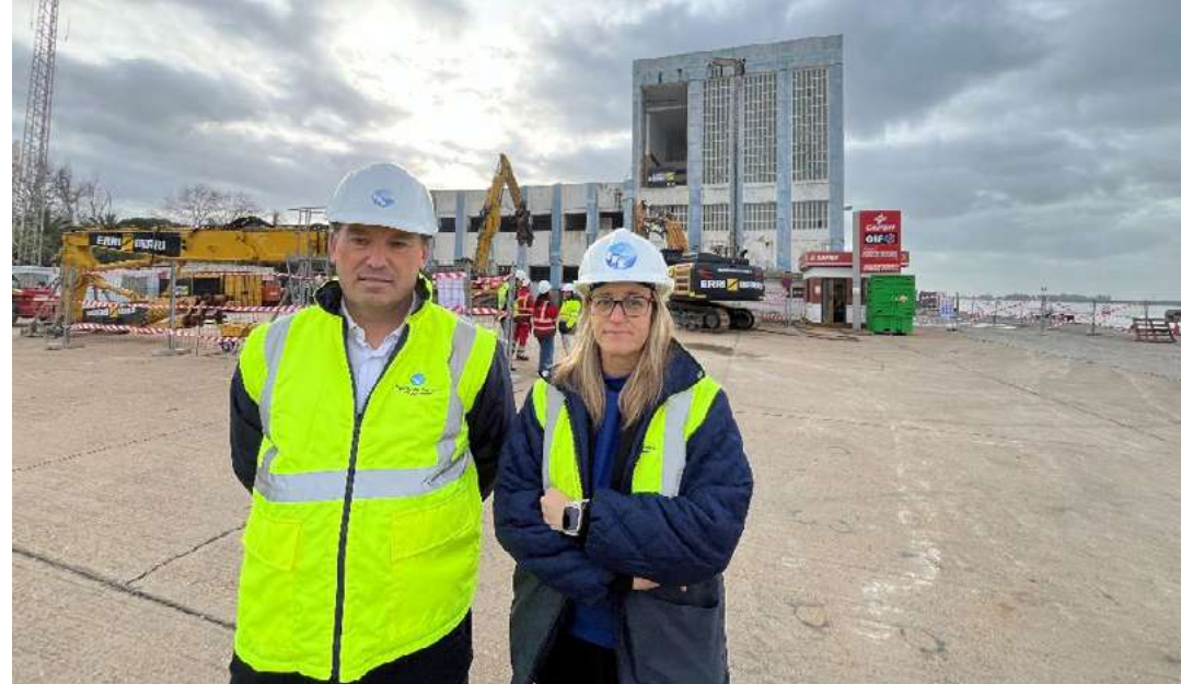
The President of the Port of Huelva, Alberto Santana, and the Head of the Infrastructure Department, Guadalupe Díaz, during the start of the demolition of the Expofrisa warehouses.
